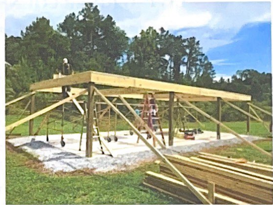
Parks' Park Pavilion being constructed with volunteer labor coordinated by Charlie Durham. This pavilion was made possible by a gift from Sam and Virginia Parks of First, Tuscaloosa.
